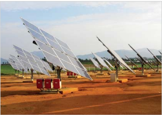
Gochang Solar Plant
