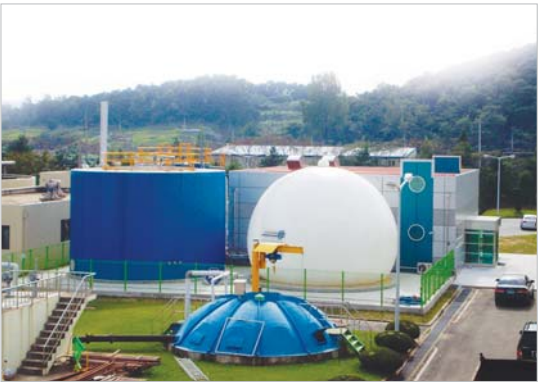
Asan intergrated type Biogas facility
