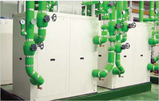
Geothermal heat pump in Namyangju
