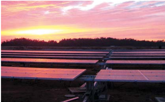
Shinan Solar power plant
