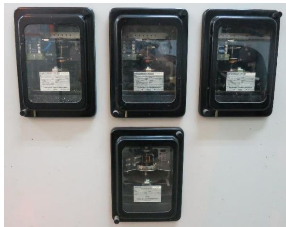
Figure 44. Over Current Relay for Distribution Feeder.
