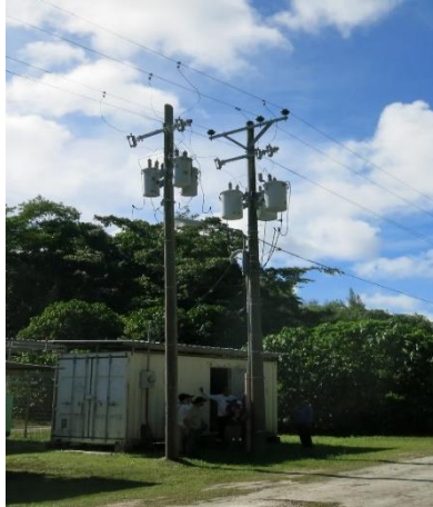
Figure 18. Pole Transformer from PV to Grid.
